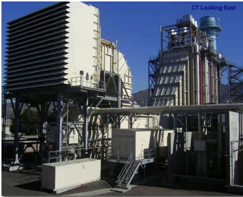
Magnolia Power Project
